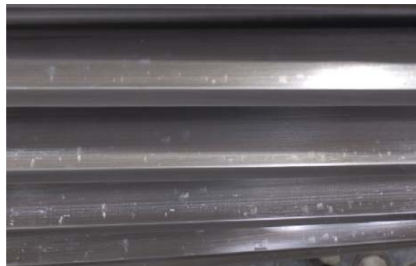
Figure 1c. Foreign object debris (FOD) damage
